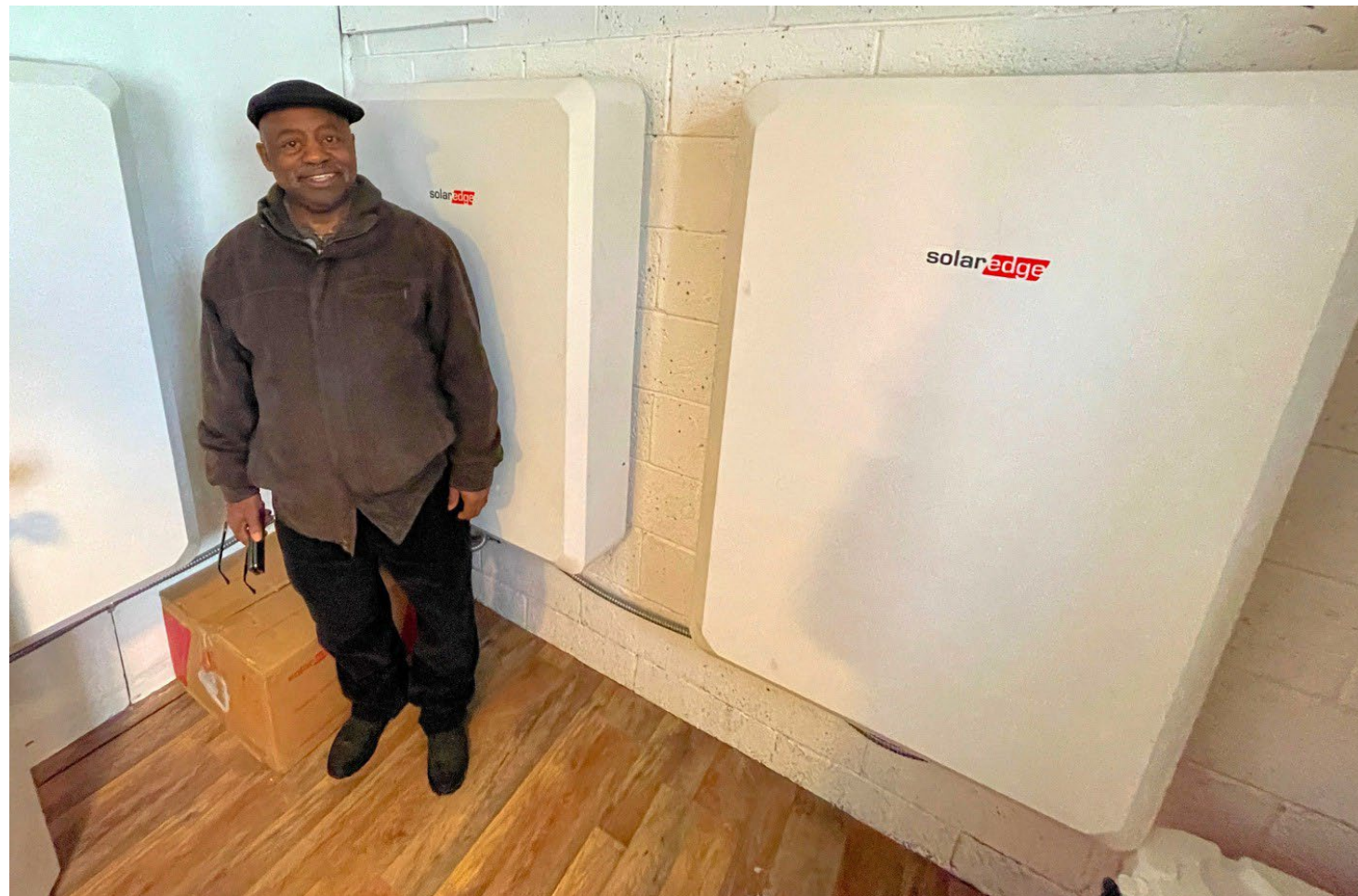
Batteries installed at Lord of Lords church in Detroit
