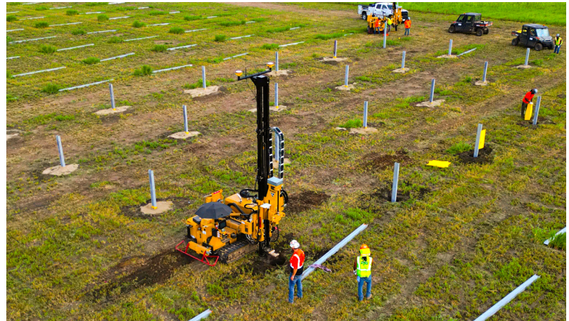
The LiveWire Energy Team working on a 7 MW solar project in McLean County, Illinois. Photo courtesy of LiveWire Construction.
